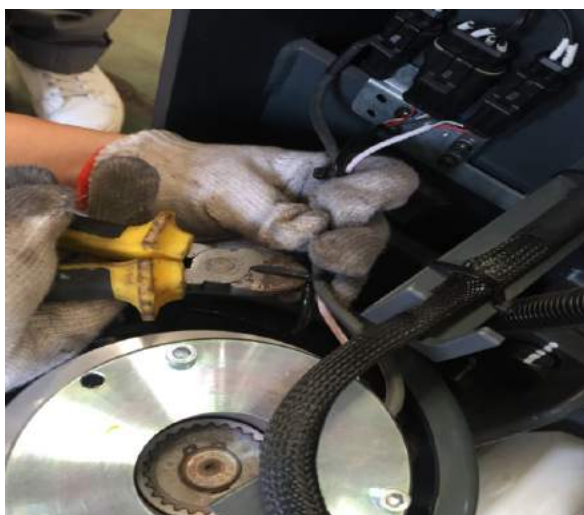
6. Use diagonal pliers to cut the tie that binds the wire harness.
